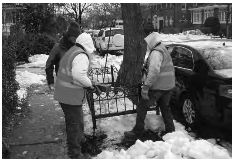
After years of waiting, Midwood and Maple are finally getting their long-awaited tree guards. Crews began the installation about two weeks after the first blizzard. photo: Ben Edwards
